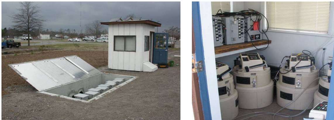
Figure 4. Monitoring vault and shed (left) with detail of sampling equipment (right)
